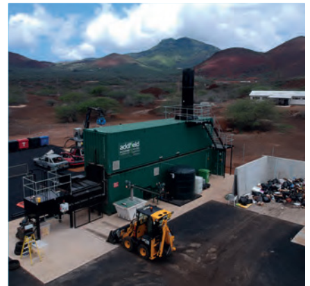
Containerised Treatment Facility Ascension Islands
